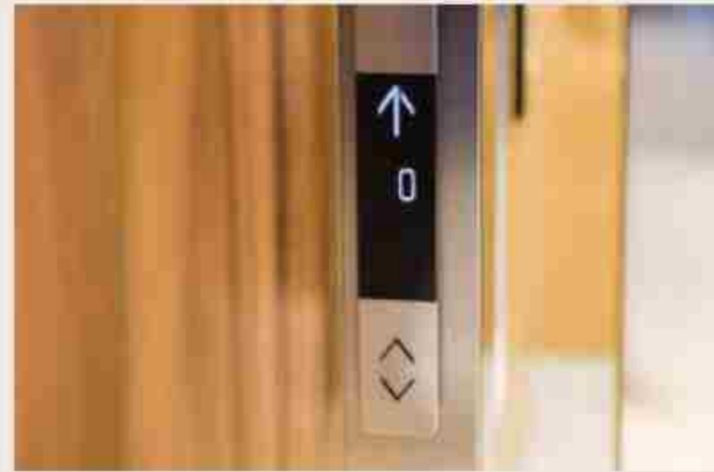
Elevator in each mansion
